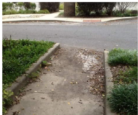
Accumulation of dirt and debris may be evidence ponding is occurring at this ramp.
