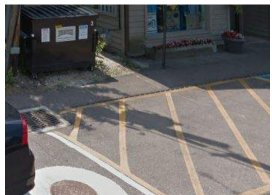
Non-compliant inlet and trench drain castings are located within a sidewalk and accessible parking space
