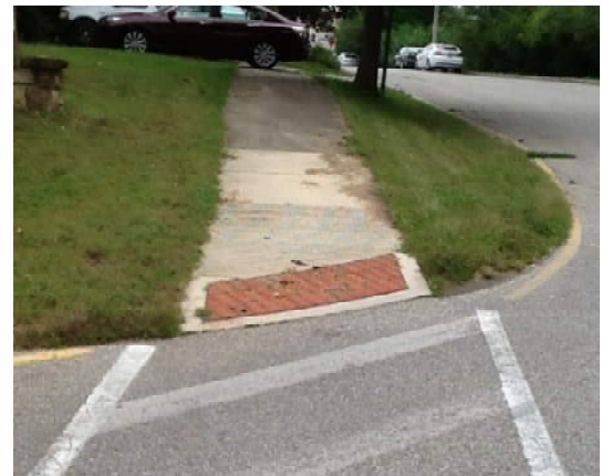
Cross slope of a ramp may be impacted by the grade found where it meets the roadway.
