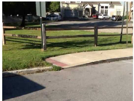
Ramp does not provide bottom turning space. Turning on steep slopes can create an unstable condition for persons with mobility devices.
