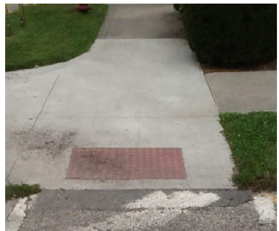
Example of detectable warning that does not extend full width of curb ramp
