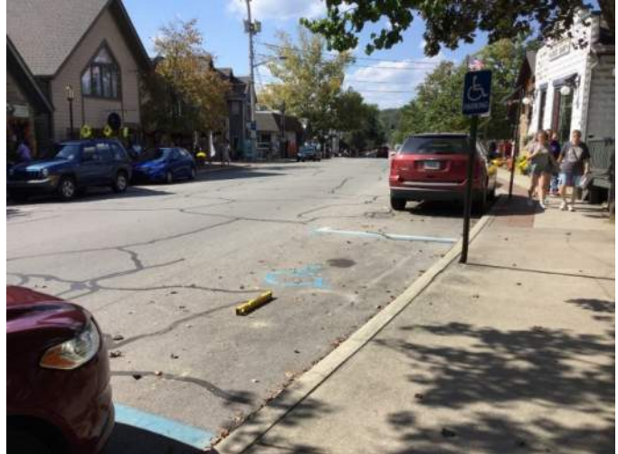
Accessible signage is provided at several designated parking spaces, but not all are located at correct heights or relative to the parking space.
