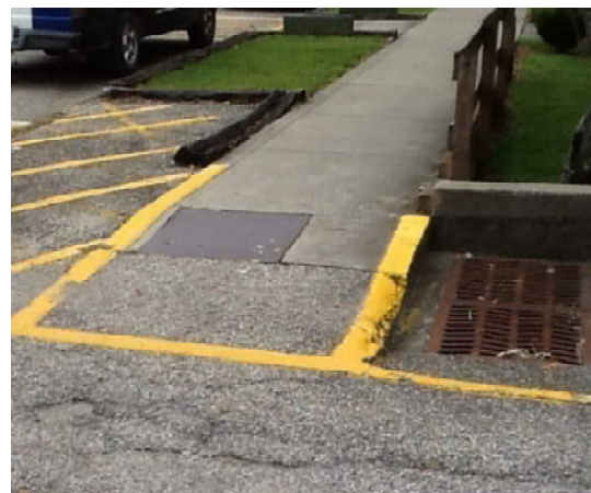
Ramp is adjacent to drainage structure which may create an issue with access during rain events.
