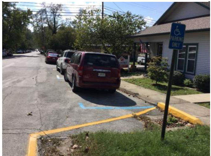
Accessible parking was frequently not located adjacent to a compliant curb ramp.
