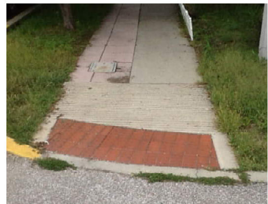
Flares are not required where lawn is provided on both sides of a ramp.
