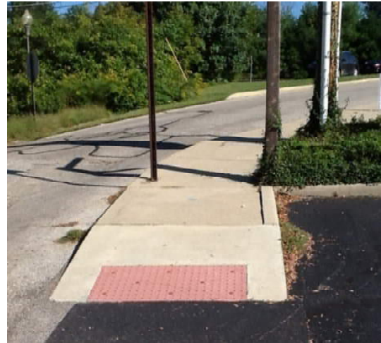
Detectable warning does not extend full width of ramp nor does it meet the 2” max. border allowed in some circumstances for proper installation of products.
